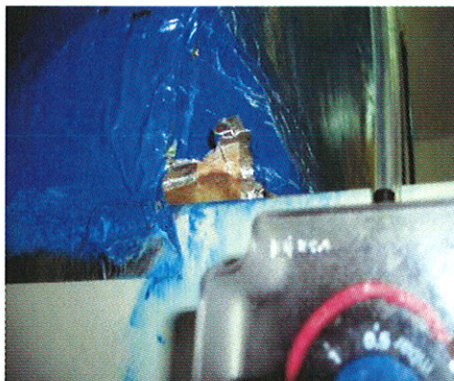
Photo A3-29 Insulating material for air conditioning system, Plant Room
