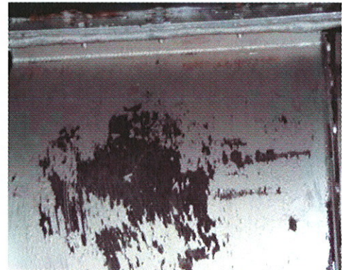
Photo A3-30 Flexible joint, I.D. Fan
