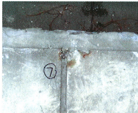
Photo A3-4 Concrete tiles, Roof of coffin crematorium building (Sample No. B/261/06/7)
