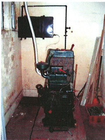
Photo A3-59 Switch Room in Skeletal Cremator Building
