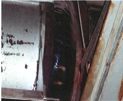
Photo A3-31 Flexible joint, Cremator Room
